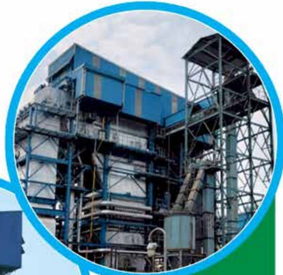
45 TPH Biomass Briquette fired Boiler at Godrej Industries Ltd. Valia (Gujarat)
