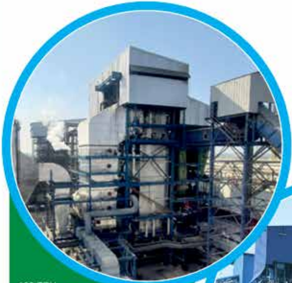
100 TPH Biomass including 70% Bagasse Pith fired Travelling Grate Boiler at Bindal Papers Ltd. (Sugar Division), Bijnor (U.P.)
