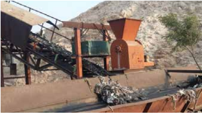
RDF feeding conveyor system
